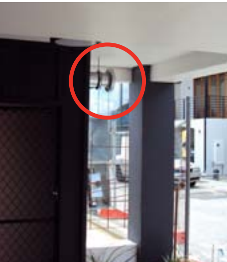
Flue terminal circled in red above
